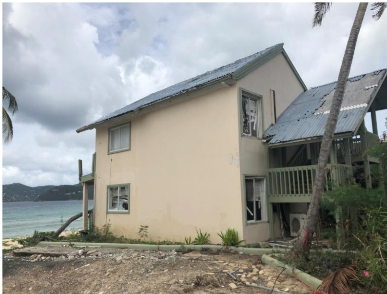
The devastation of Hurricane Irma took many of the resort's facilities offline, including the wastewater plant.
